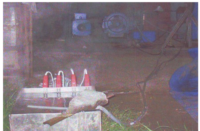
Fig. 5 . Installation of Diesel Engine with Electrical Loads
