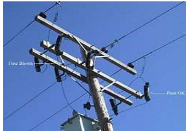
Fig. 4. Transmission Line One Side Fuse Blown & Other Side Fuse Is Ok
