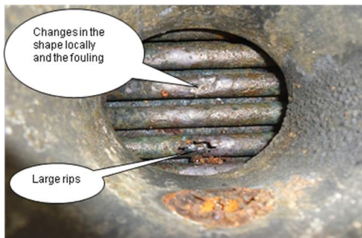
Fig. 1.3. Photos of the damaged tube [2]
