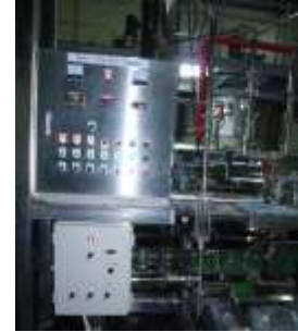
b) Control panel
