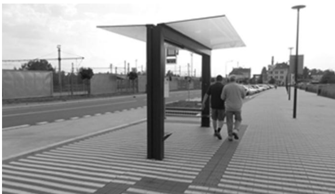
Fig. 8 Unsuitable location of the stop roof.
