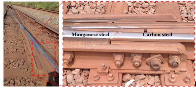
Fig. 8. (a) Turnout overview, highlighting the heel; (b) transition between manganese and carbon steel
